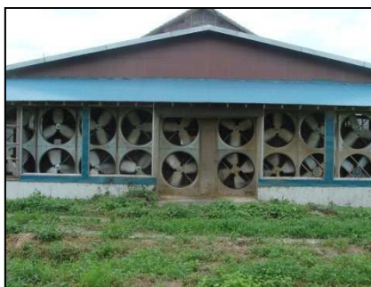
↑牛舎壁面の換気扇
